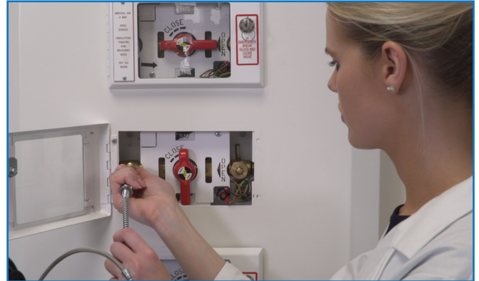
Direct connection to any terminal unit or NIST through a robust stainless-steel braided hose.
